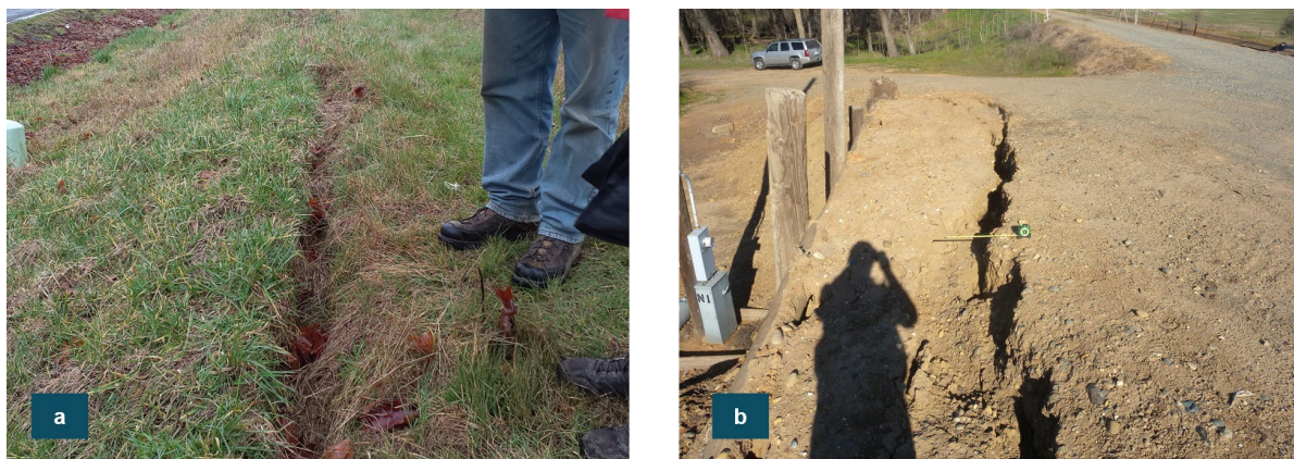
Figure 9-10: Example of Tension Cracks
