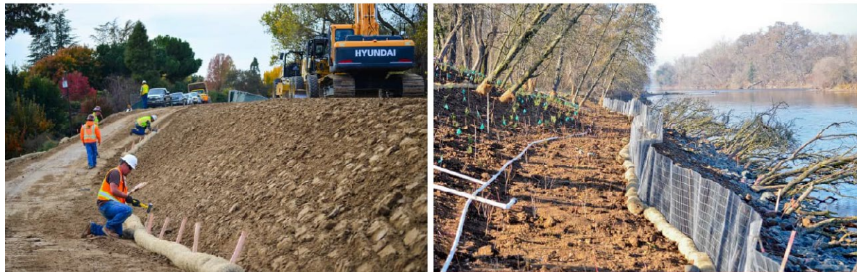
Workers install straw wattles (left) and silt fences (right) along a new American River levee section in the River Park neighborhood of Sacramento California; November 2014.
