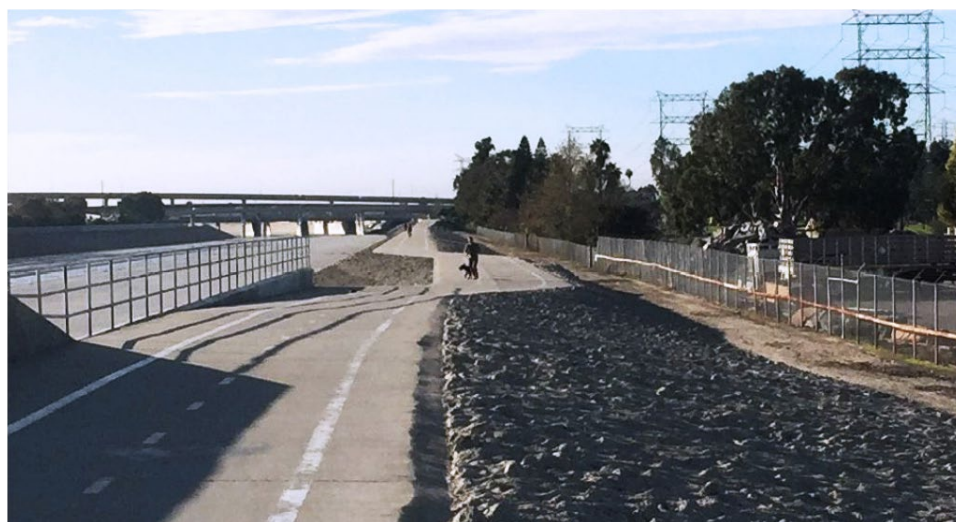
This is an overtopping section along the Los Angeles River.
