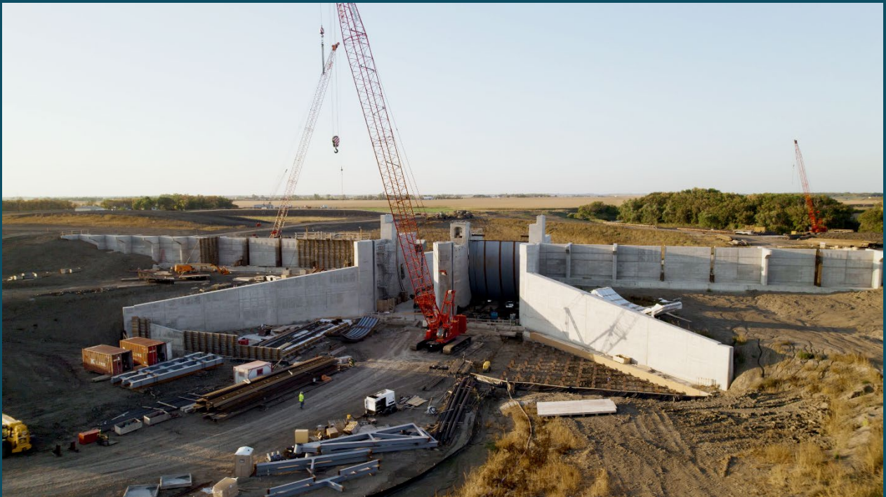
The Wild Rice River structure being built as part of the Fargo-Moorhead Metropolitan Area Flood Risk Management project, designed and constructed by USACE (Metro Flood Diversion Authority, 2023).
