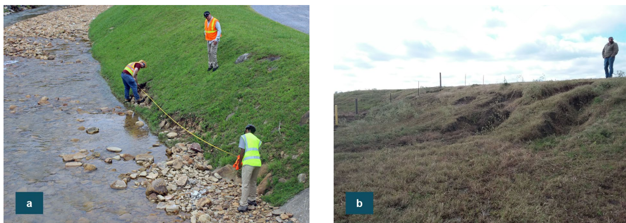
(a) Personnel measure erosion following a high-flow event along a levee in West Virginia. (b) Erosion furrows on upper slope of a levee embankment in Mississippi.
