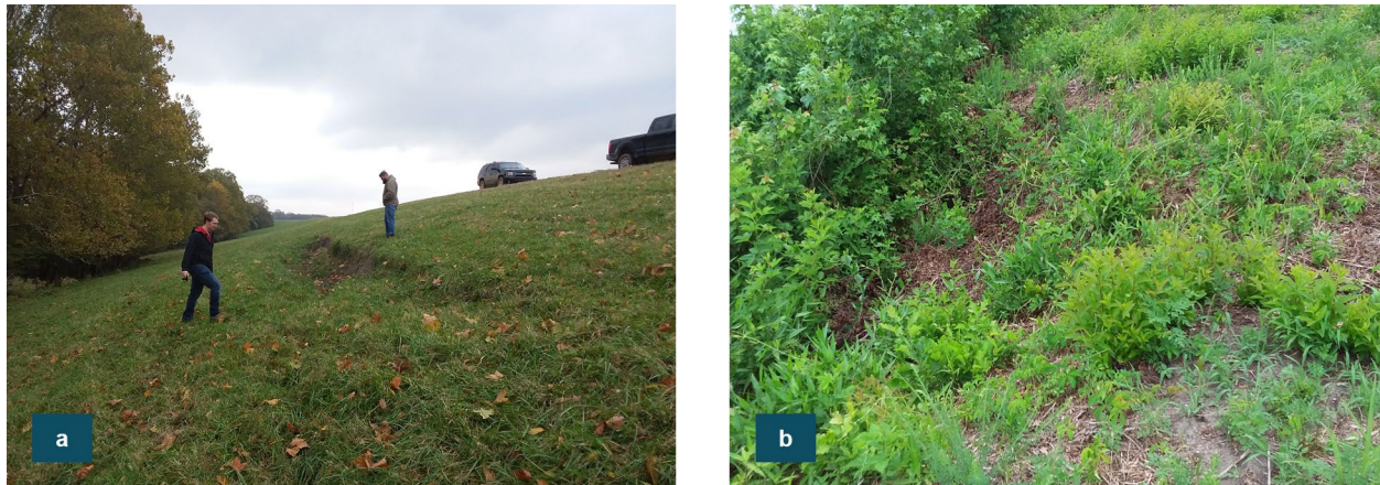
Figure 9-8: Examples of Embankment Slope Sloughs
