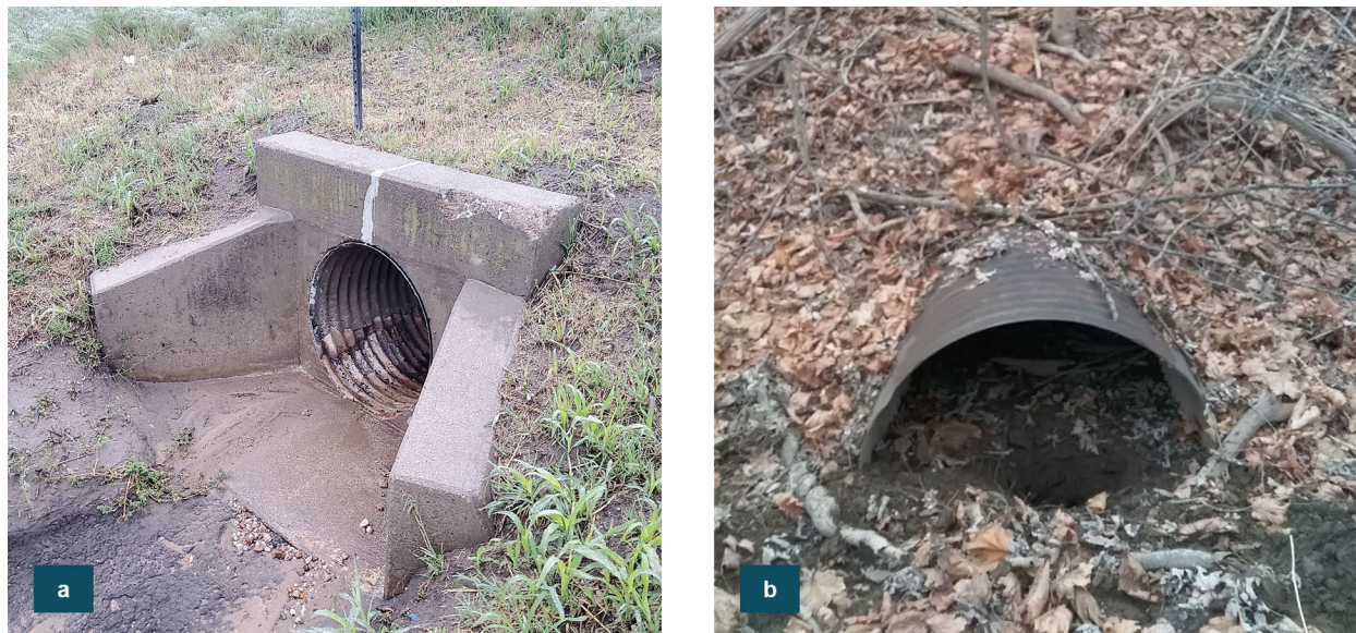
Figure 9-29: Examples of Pipe Problems
