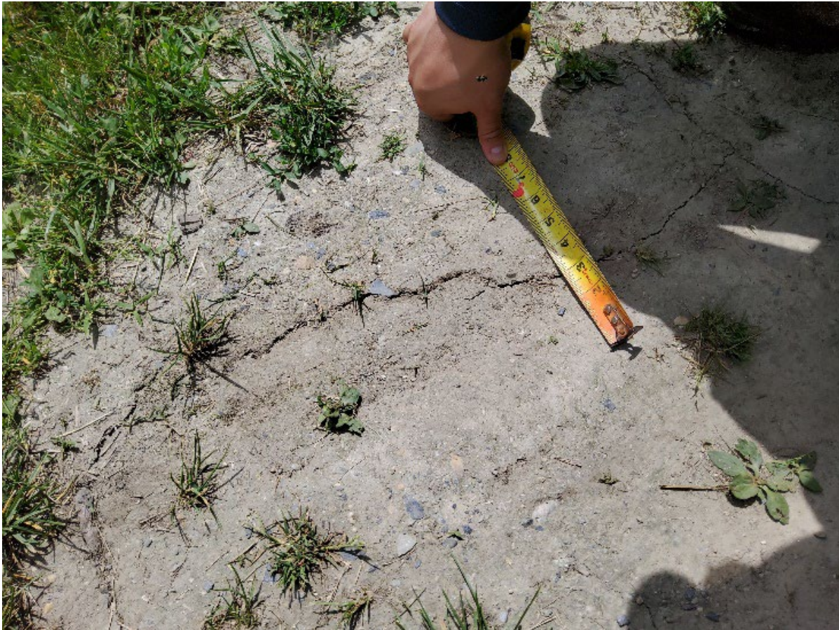
Figure 9-11: Example of Desiccation Crack
