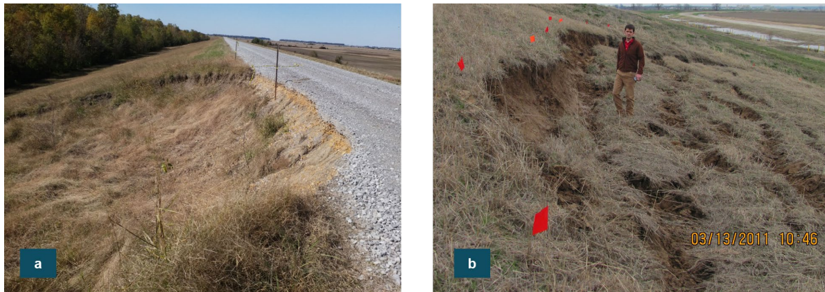
Figure 9-9: Examples of Embankment Slope Slides
