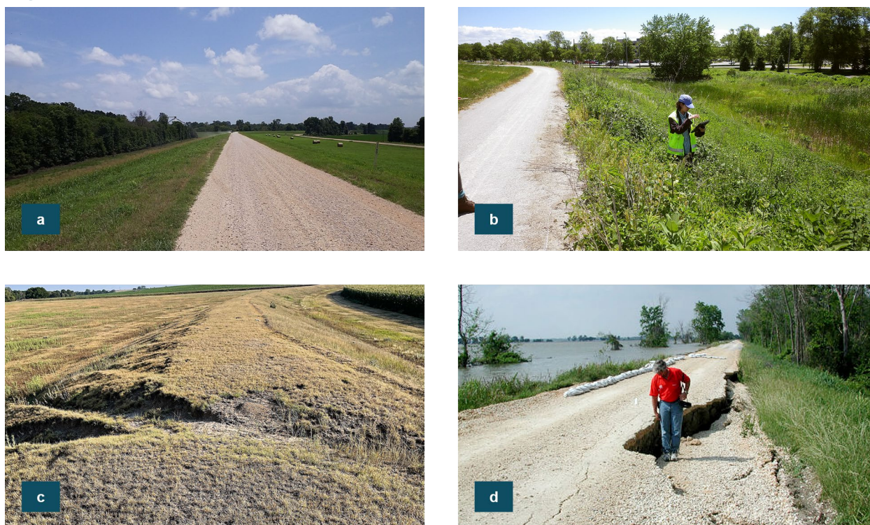
Figure 9-5: Examples of Levee Maintenance Conditions
