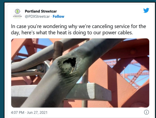
Heat damage to a power cable.
