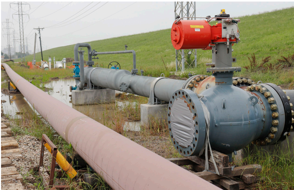
Figure 7-13: Example of Utilities in the Project Area
