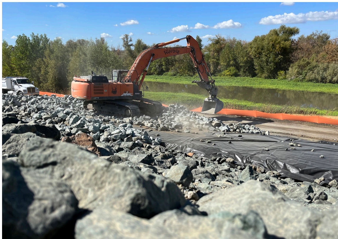
Workers install riprap erosion protection along a levee in West Sacramento, California; September 2023.
