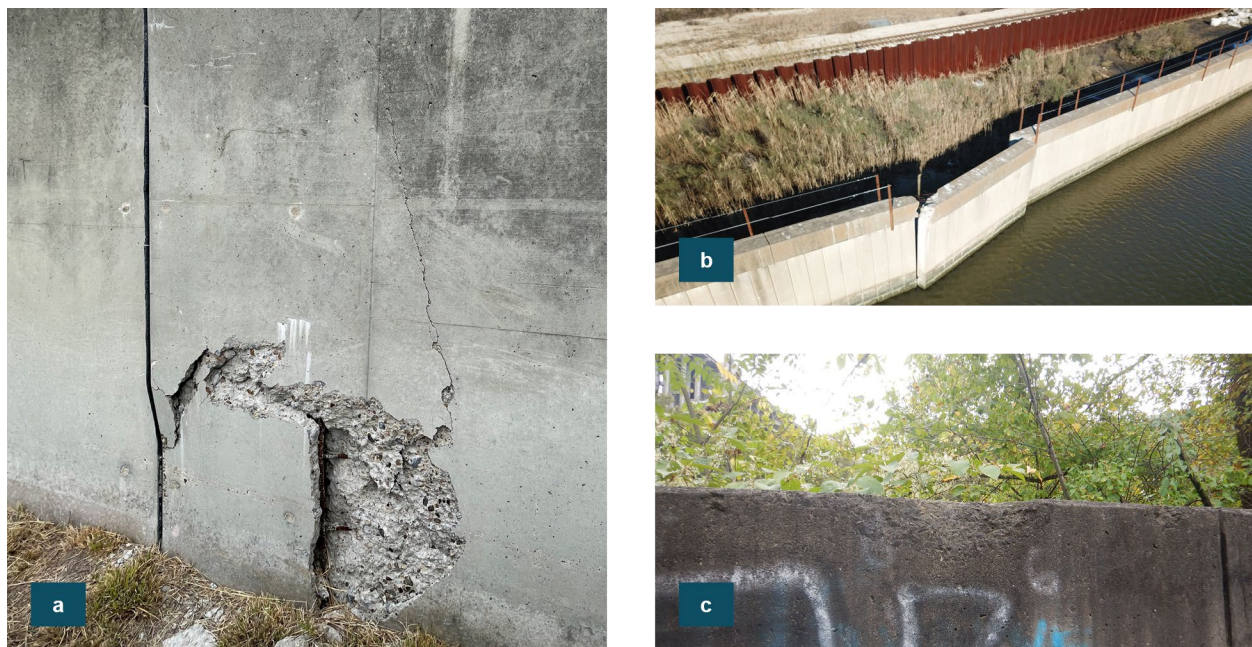
Figure 9-21: Examples of Floodwall Damage
