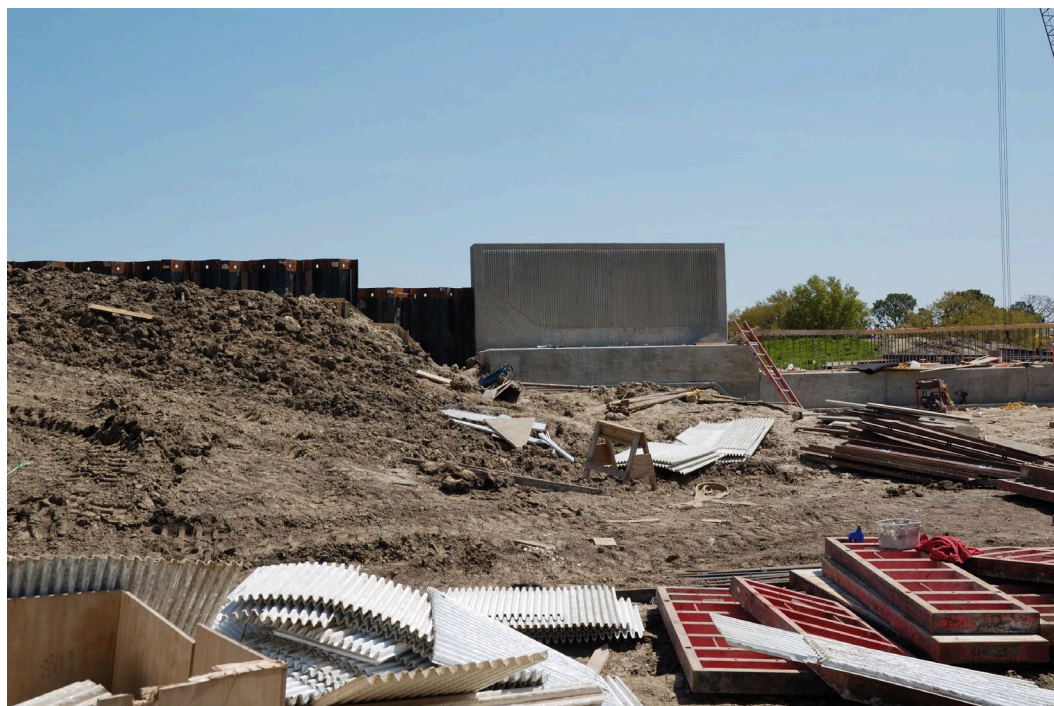
T-wall to I-wall to embankment transition under construction in New Orleans, Louisiana.
