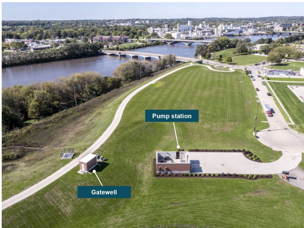
Interior drainage system showing the pump station and gate house on a levee in Cedar Rapids, Iowa.
