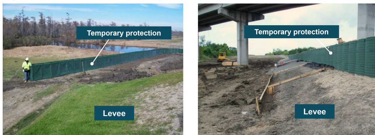
Figure 7-8: Examples of Temporary Flood Protection
