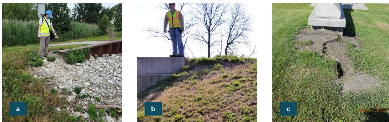
Figure 9-26: Examples of Transition Zone Damage
