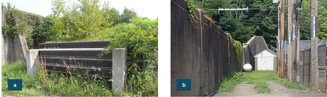
Figure 9-22: Vegetation Impacting Floodwalls
