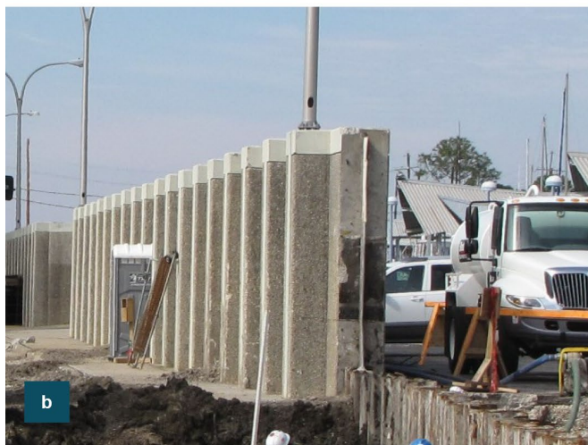
(a) L-wall being constructed in St. Louis, Missouri. (b) I-wall being constructed in New Orleans, Louisiana. (c) T-wall being constructed in New Orleans, Louisiana.
