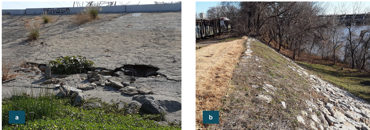
Figure 9-16: Examples of Damaged Slope and Bank Erosion Protection
