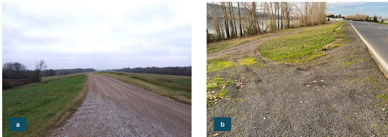
Figure 9-17: Examples of Levee Roads Needing Repair
