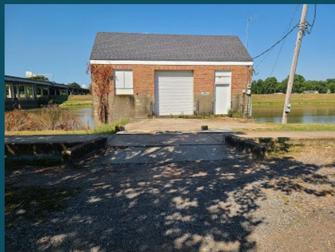
The condition of the Calypso Street pump station prior to repairs beginning.
