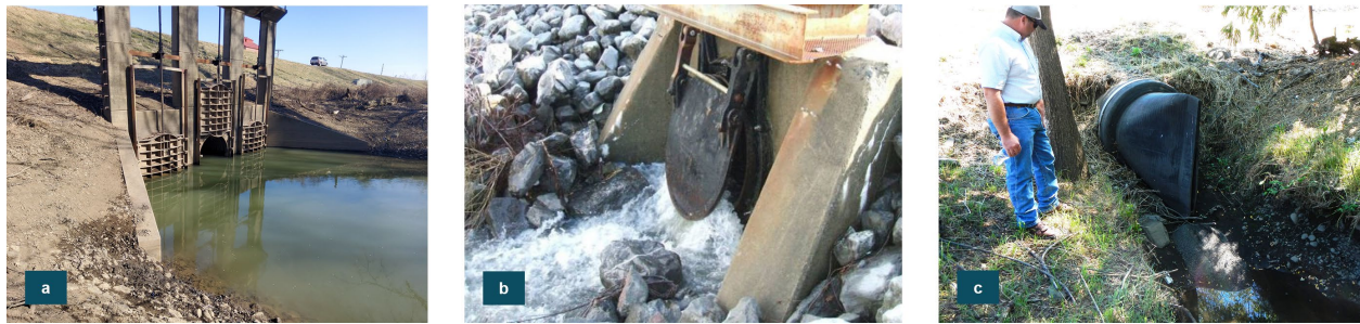
(a) Sluice gate being used for interior drainage. (b) Use of a flap gate for interior drainage. (c) Duckbill being used for interior drainage.
