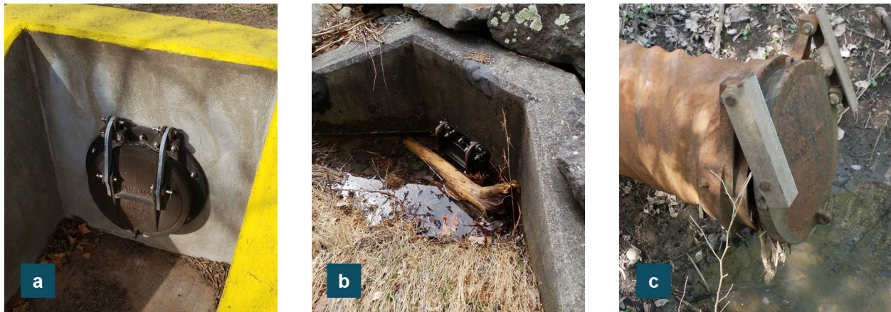
Figure 9-32: Examples of Flap Gate Condition
